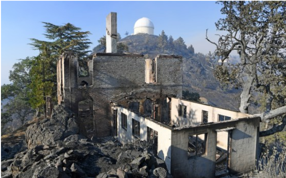
A Lick Observatory building destroyed by the SCU Lightning Complex Fire atop Mount Hamilton, Calif., on Thursday, Aug. 20, 2020. (Doug Duran/Bay Area News Group)
